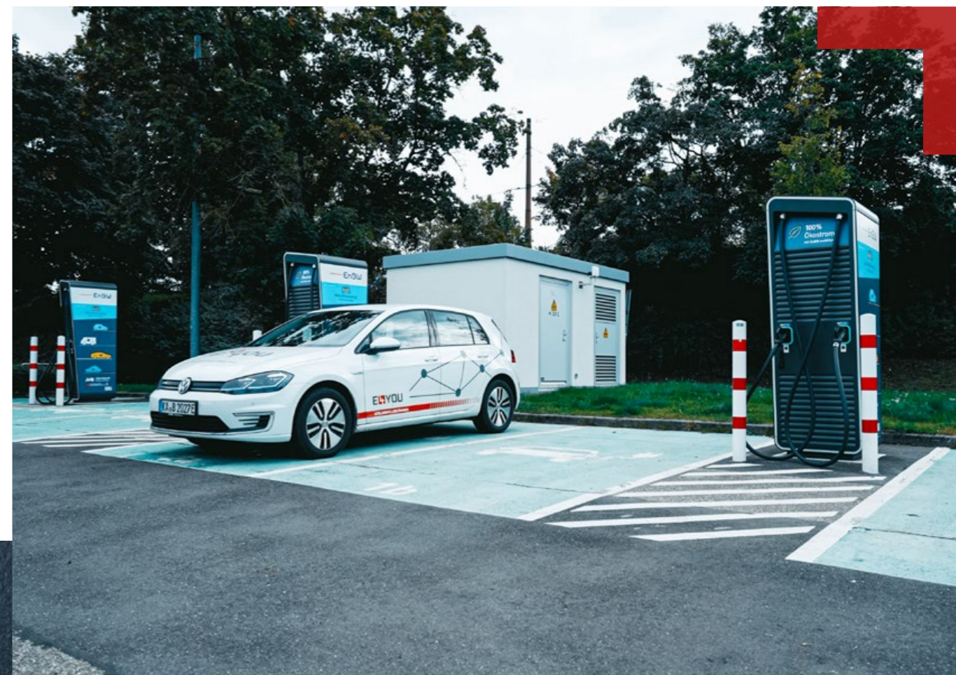
Compact Substation in public area for supplying electricity to a charging point
